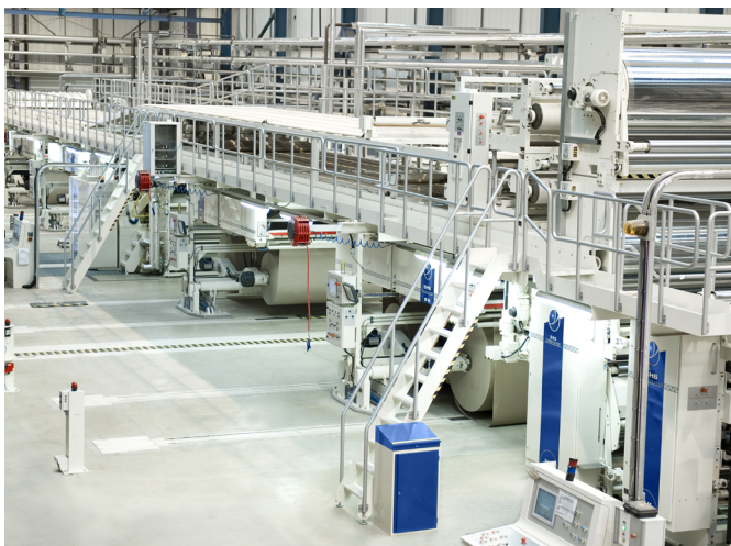
BHS Corrugated Wet End
